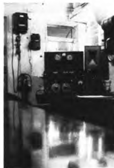
SS.South American - WGCW Emergency spark Xmtr on fwd bulkhead, top right.
